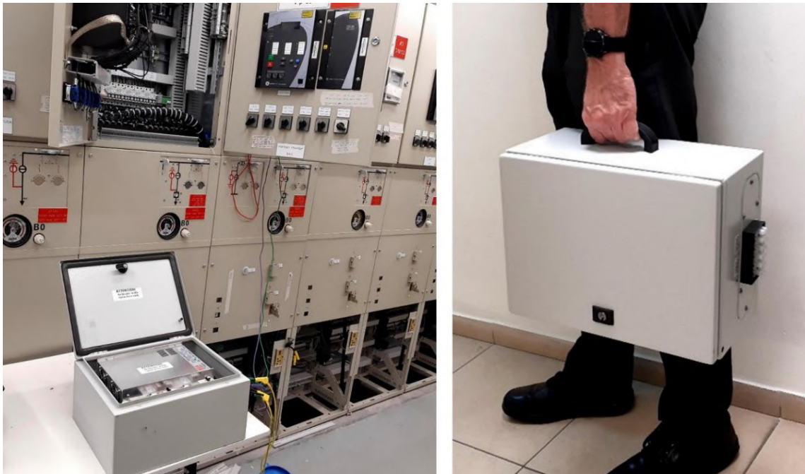
Fig. 22. HEMP protected backup power supply for electronic equipment testing after HEMP impact
