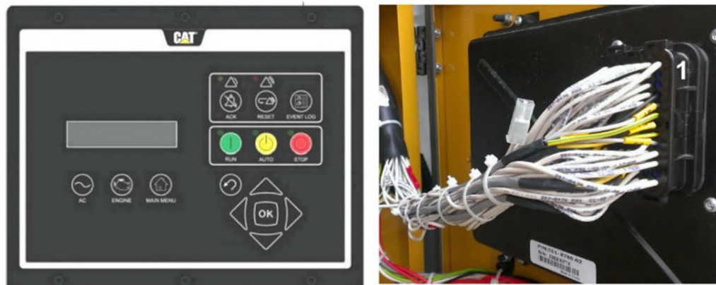
Fig. 26. Main controller of diesel generator
