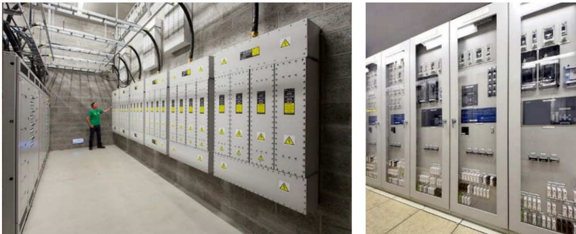
Fig. 6. HEMP filters (left) and control cabinets (right). For size comparison.
