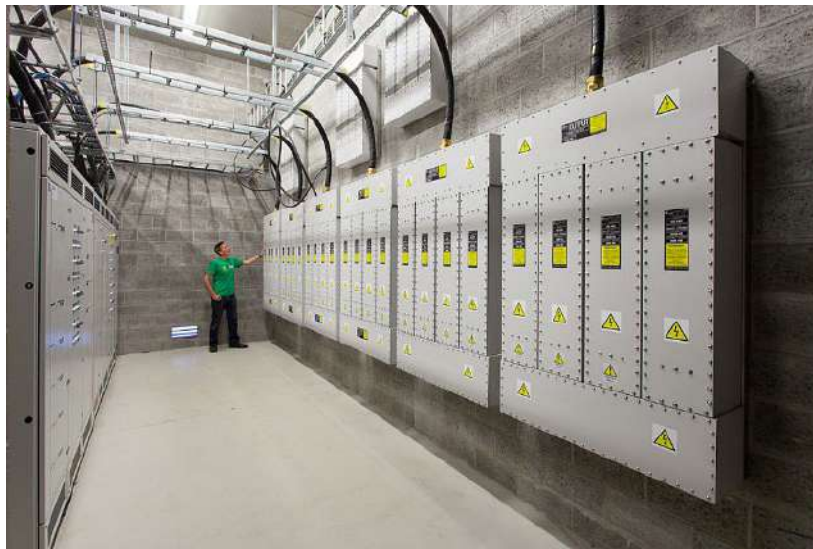
Fig. 3.8. HEMP filters installed in a military bunker protected against the nuclear explosion.
