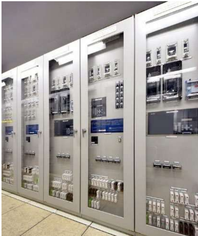
Fig. 4.1. Electronic equipment controls cabinets used in the power industry
